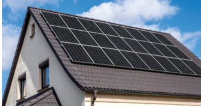
Solar PV System
